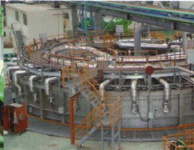
▲ Rotary Heating Furnace
